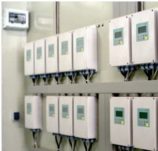
Primärkühler Analysenteil Messumformer Primary Sample cooler Analysing equipment Transmitter
